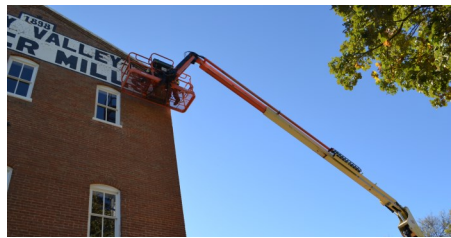
Local company Perfect Blend completed tuckpoint masonry repair to the Old Mill exterior brick.
